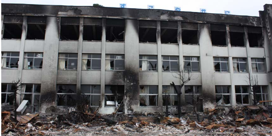
Fig.30 Burn mark of pattern-2 automobile fires at the wall of Kadonowaki elementary school building. ( Kadonowaki district in Ishinomaki city, Miyagi prefecture, photo taken on 11 th April 2011 )
