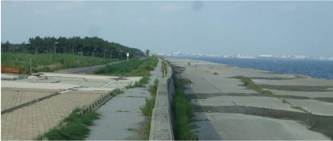
Fig. 8. Seawall pushed forward (Photo taken on Aug. 1 st , 2011 at 35.63666, 139.931638)
