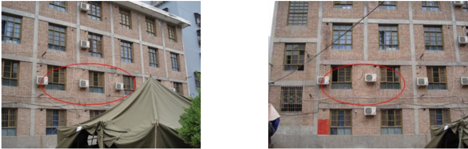
Fig.5 The building with improper force transmission path
