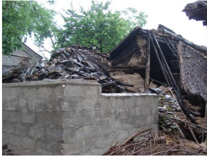
Fig.2 The collapsed timberwork buildings
