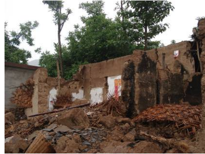
Fig.3 The collapsed raw-soil structure buildings
