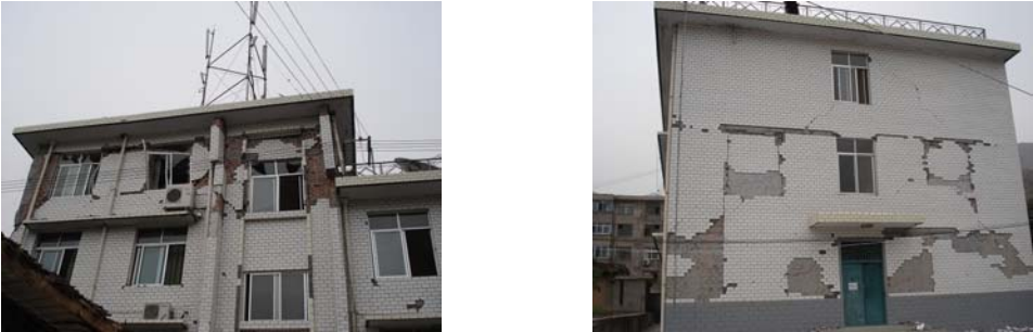
Fig.6 the damages of Meteorological Bureau building in gansu province
