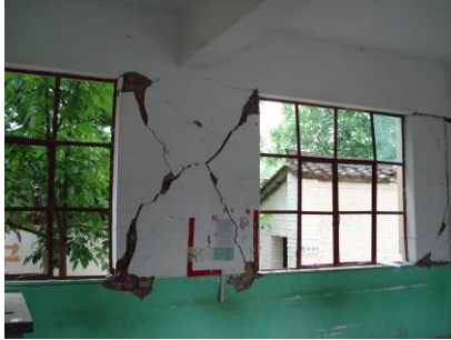
Fig.9 The ‘X’ form shear cracks of vertical wall
