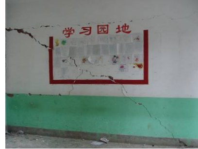
Fig.10 The diagonal cracks of cross wall
