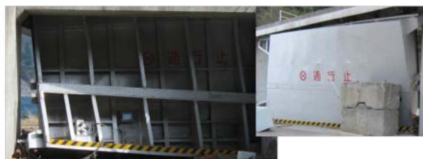
(a) Destroyed sea wall gate (Miyako)
