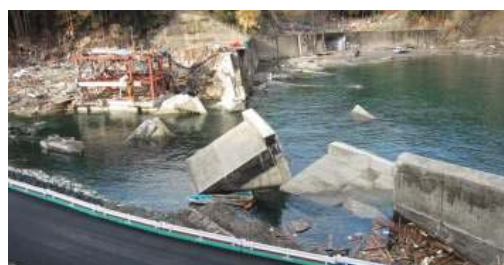
Photo 4 Seawalls toppled due to scouring (Ryou-ishi, Miyako)
