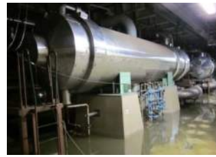
Photo 6 Heat exchanger room at Onagawa NPS RB basement (by Tohoku EPCO)
