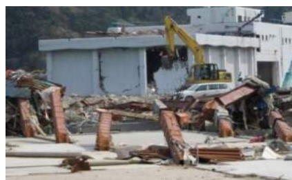
(b) Bent steel pillars (Onagawa)
