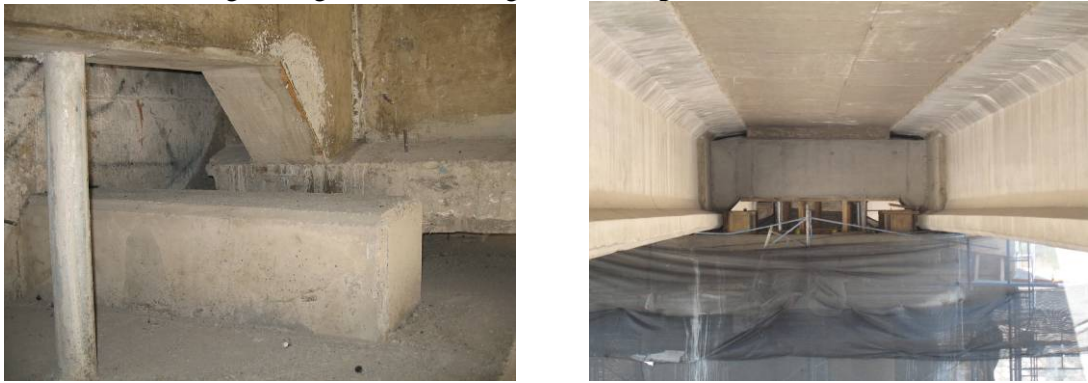
Photo 9 Repair and Retrofit for Les Mercedes Bridge (2) (Left: Lateral Stopper at Abutment, Right: Lateral Beams and Lateral Stoppers at Pier)
