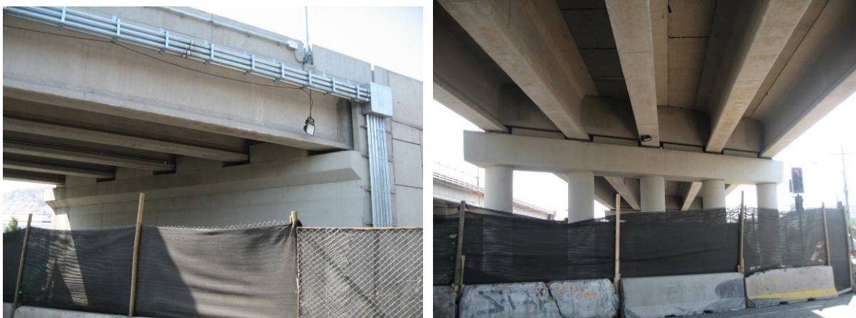
Photo 4 Repair and Retrofit for Lo Echeveres Overpass (Left: Lateral Stopper at Abutment, Right: Lateral Beam and Lateral Stopper at Pier)
