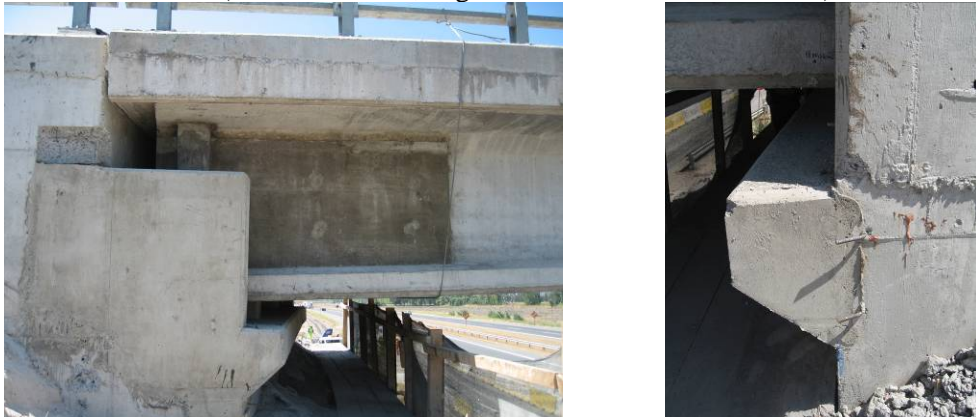
Photo 8 Repair and Retrofit for Les Mercedes Bridge (1) (Left: Strengthening of PC Web, Right: Widening of Seat Width at Abutment)
