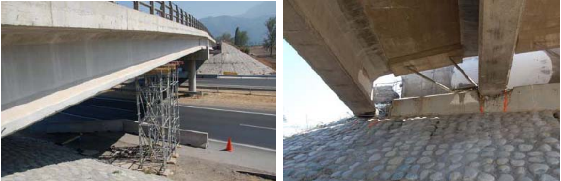
Photo 7 Damage of Les Mercedes Bridge (Left: Side View, Right: Lateral Offset at Abutment)
