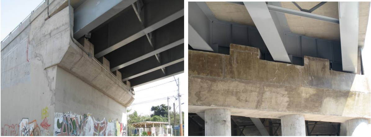
Photo 6 Repair and Retrofit for Antonio Matta Bridge (Left: Abutment with Lateral Stopper, Right: Pier Cap with Lateral Stopper)
