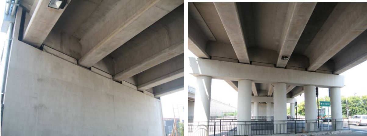
Photo 3 Repair and Retrofit for Mira Flores Overpass (Left: Lateral Stopper at Abutment, Right: Lateral Beam and Lateral Stopper at Pier)
