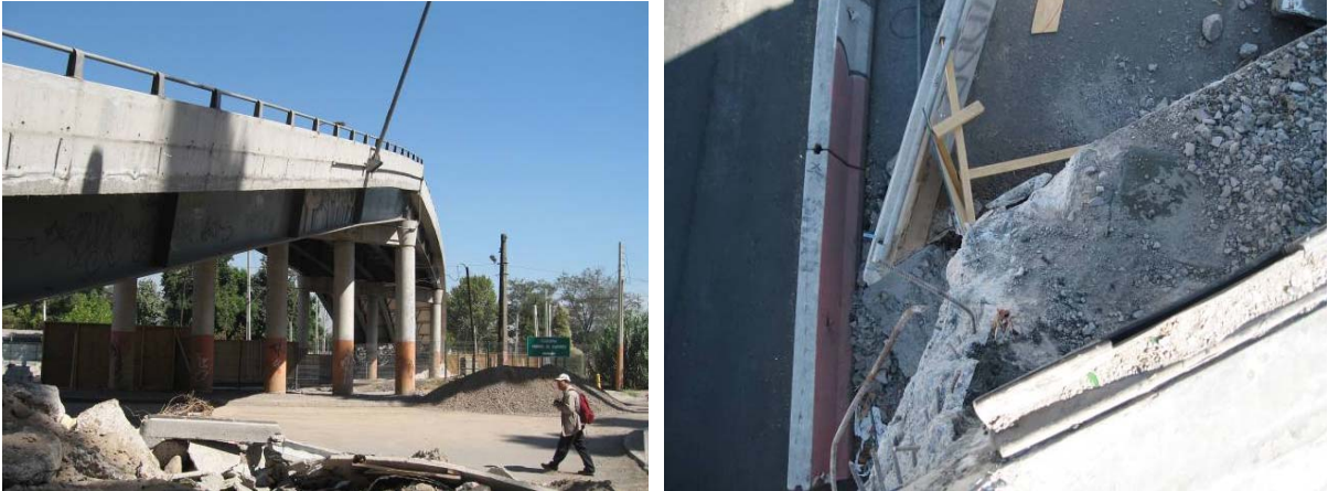
Photo 5 Collapse of Antonio Matta Bridge (Left: Side View, Right: Skewed Seat at Abutment)
