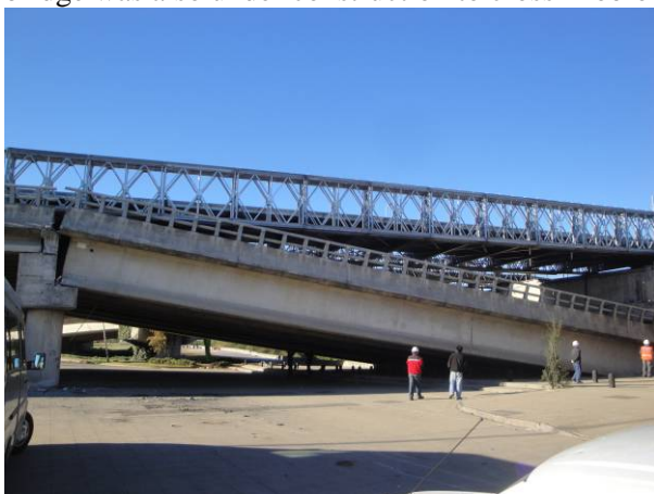
Photo 16 Collapse of Llacolen Bridge
