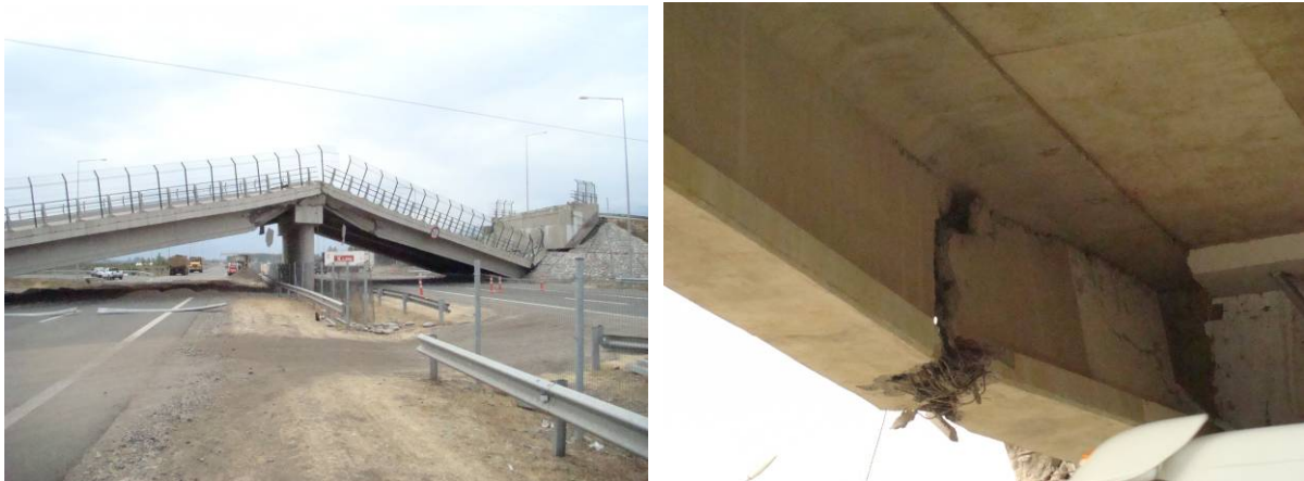
Photo 1 Typical Collapse and Damage of Concrete Girders during 2010 Chile Maule Earthquake (Courtesy of Chilean Ministry of Public Works)
