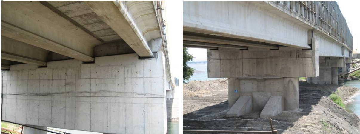
Photo 21 Repair and Retrofit for La Mochita Bridge (Left: Pier Cap with Lateral Stopper, Right: Strengthening of Foundations by Placing New Piles)
