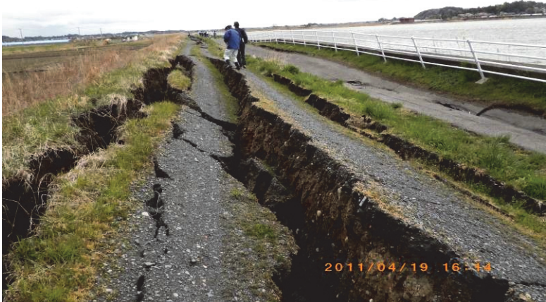
Fig. 7 Damaged levee of Hinuma in Ibaraki
