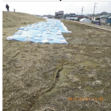
Fig. 9 Sand boils in the berm at the middle height of the Naruse River levee north of Sendai City
