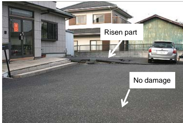
Photo 2 Upheaval of housing lot at Hebizono area
