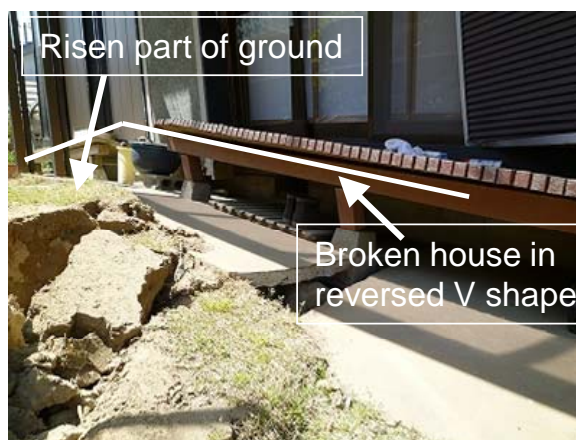
Photo 4 Destroyed house due to ground upheaval at the center of the house
