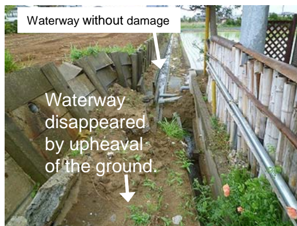
Photo 3 Boundary between unliquefied foundation and damaged foundation
