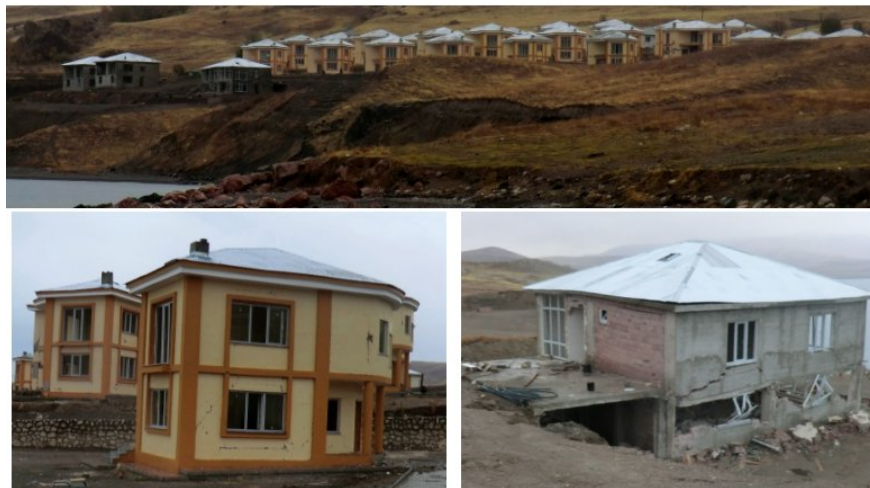
Photo 9 Damaged buildings due to permanent deformation of sloping ground
