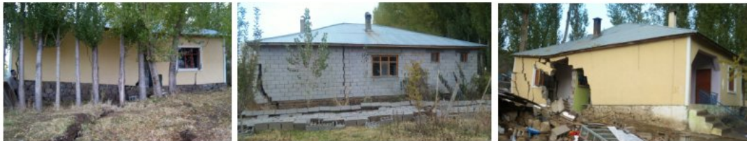
Photo 6 Lateral spreading induced damage to buildings in Çelebibağı (Erçiş)
