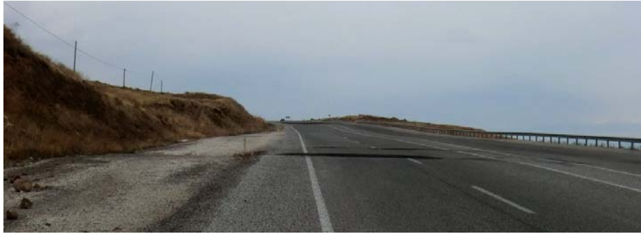
Photo 2 Embankment failure on the Van-Ağrı Highway
