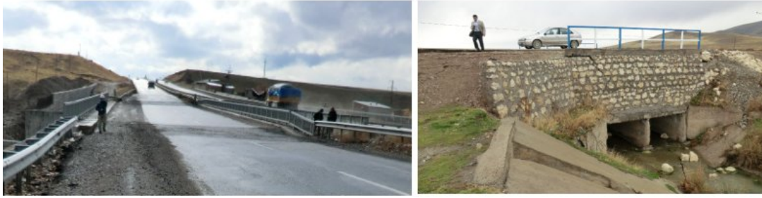
Photo 7 Damage to bridge piers and abutments due to settlement and lateral spreading of ground
