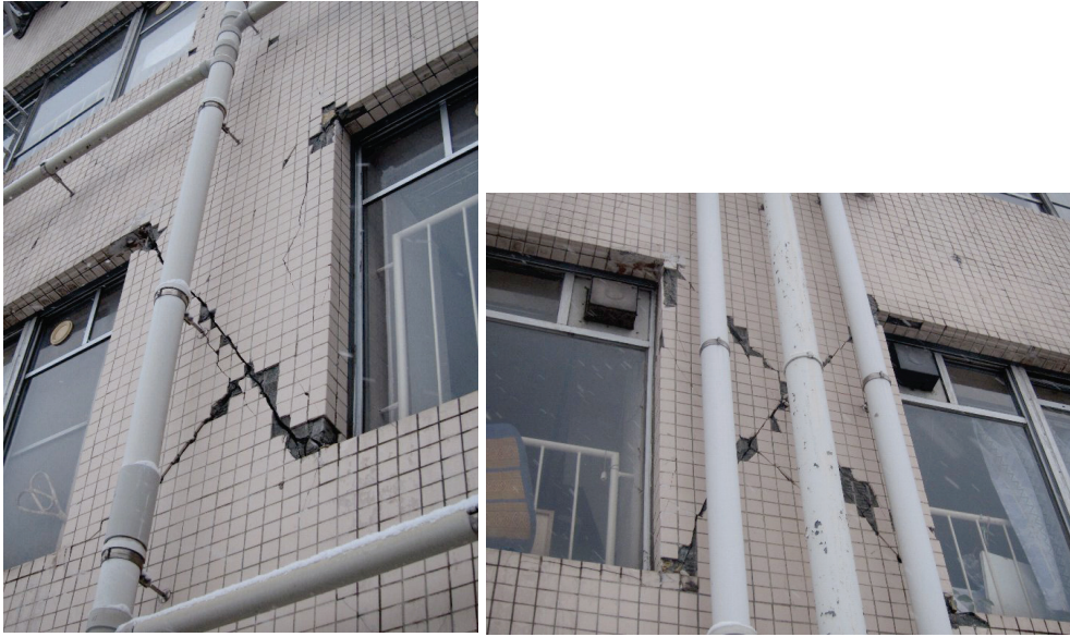
Fig. 9 Shear failure of exterior column in Y 4 frame
