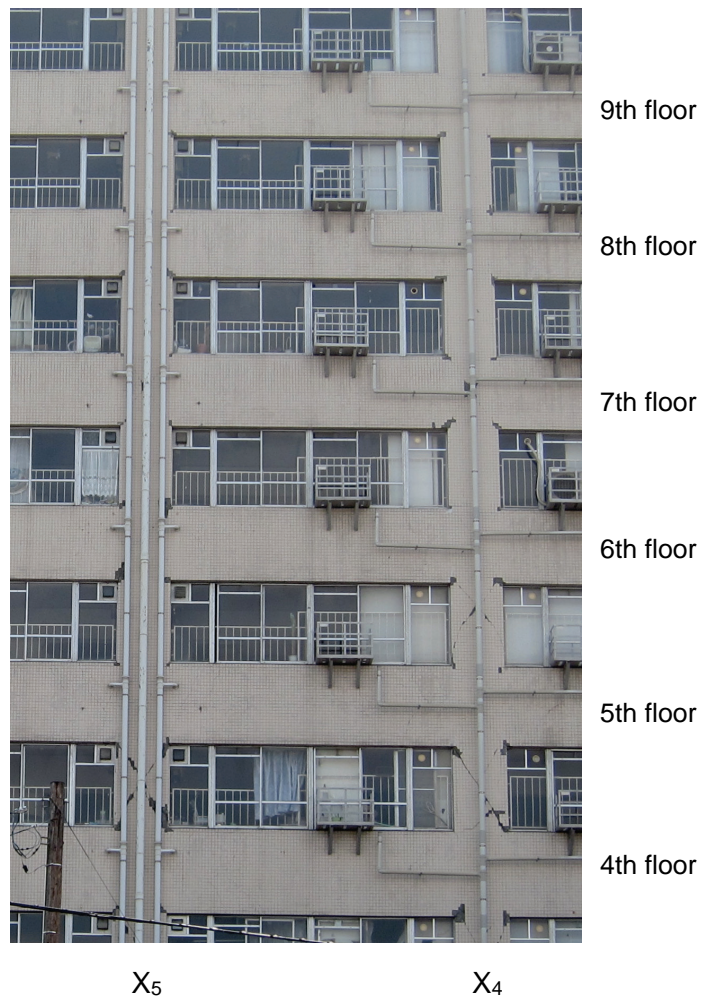
Fig. 10 Joint shear failure of beam-column joints
