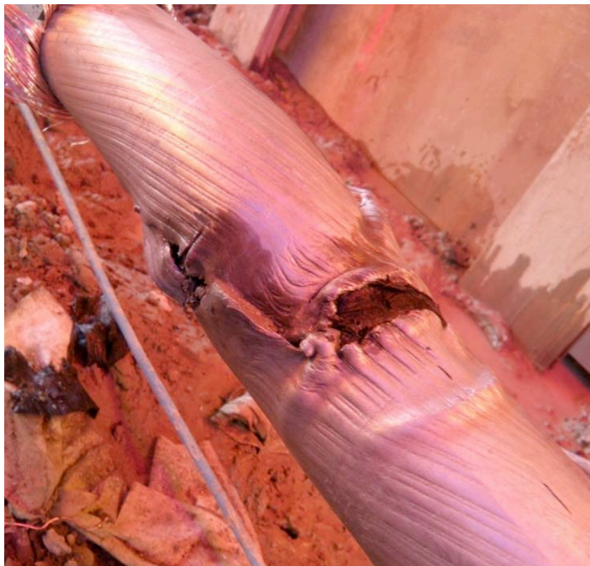
Figure 12. Failed XLPE-Type Cable, Location 4
