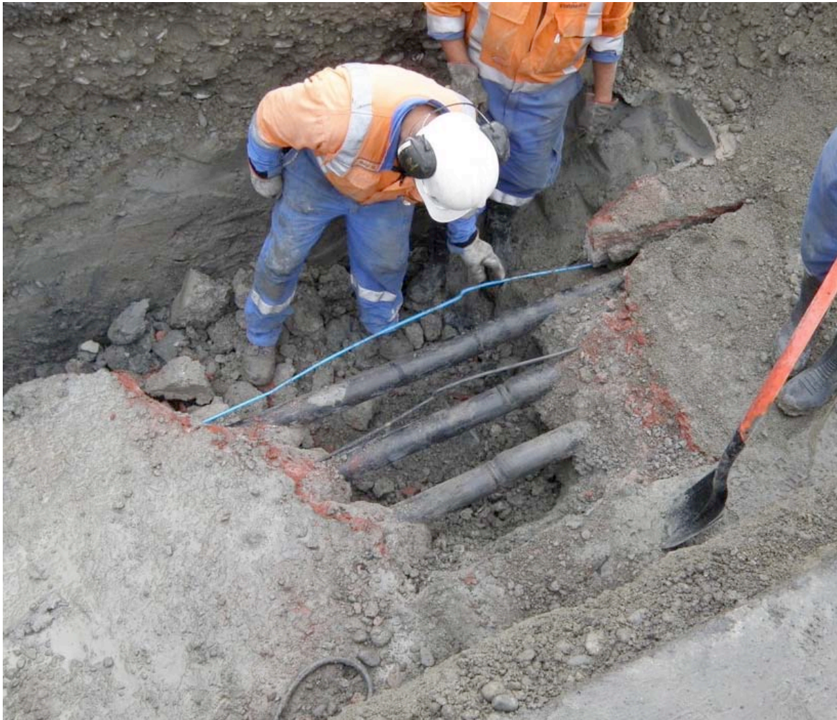
Figure 10. Exposing the Damaged XLPE-Type Cables, Location 6
