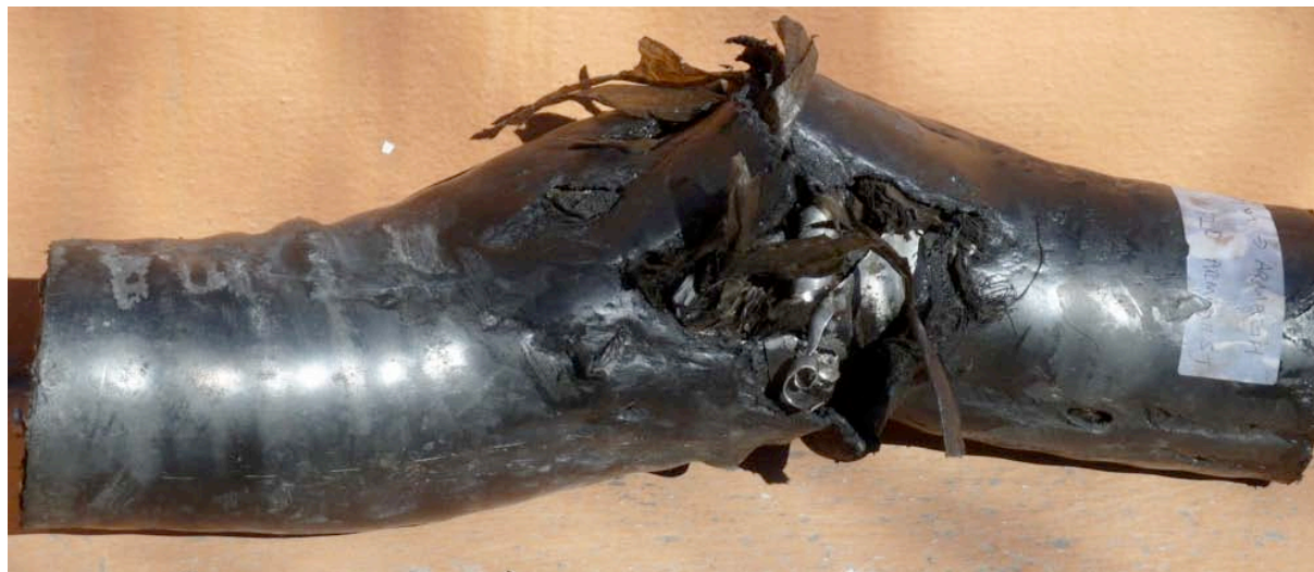
Figure 7. Oil-Type Cable (Location 3)
