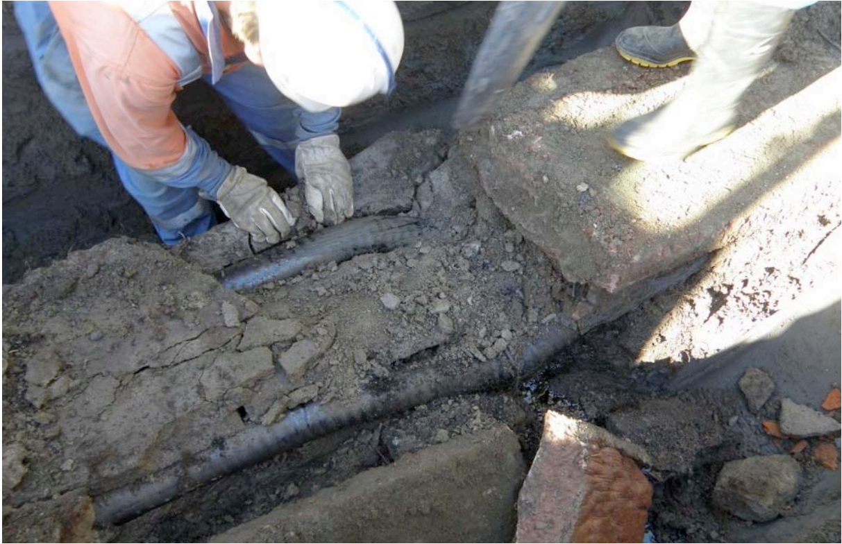
Figure 5. Exposing the Damaged Oil-Type Cables, Location 1
