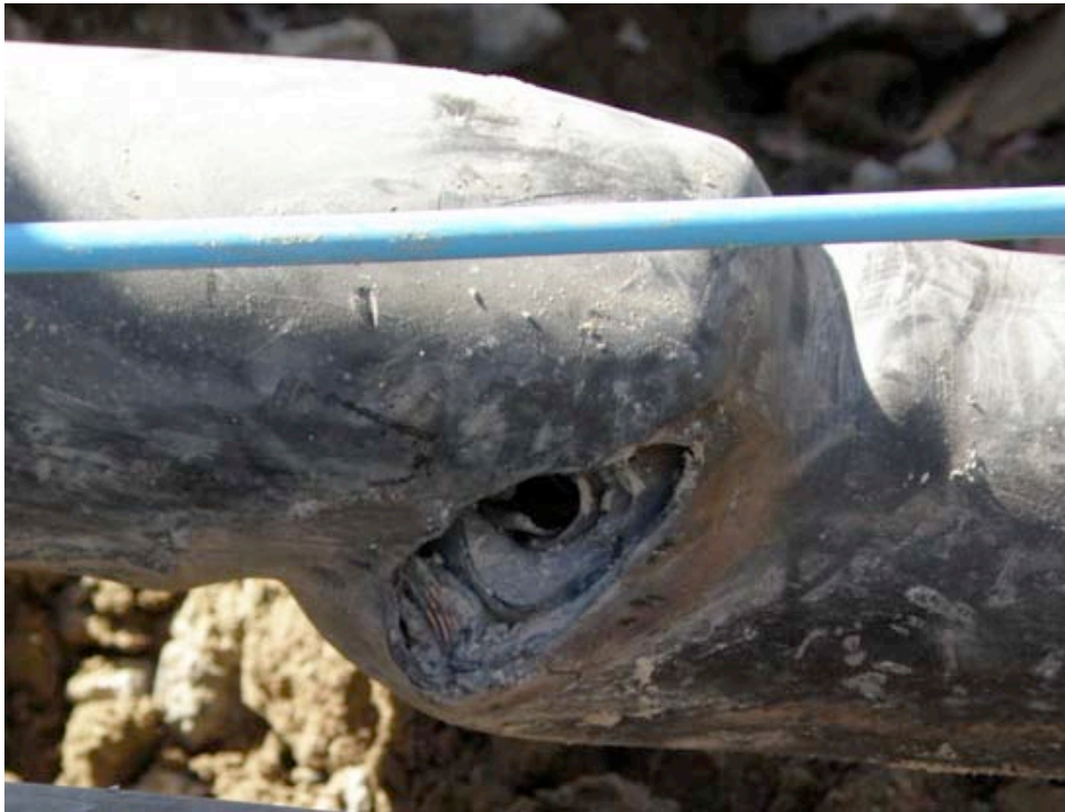
Figure 11. Failed XLPE-Type Cable, Location 4
