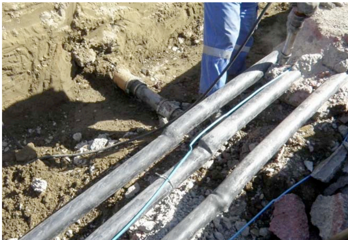
Figure 13. Failed XLPE-Type Cable, Location 5
