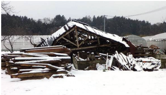
Fig. 12 Collapse of shed in Kurihara
