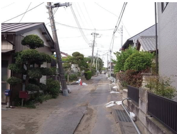
Fig.23 Damage due to liquefaction in Katori-city
