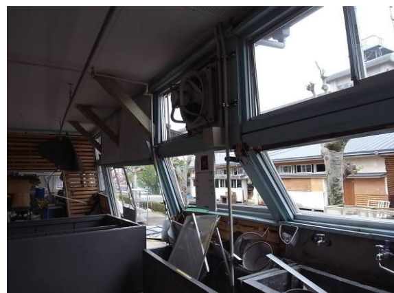
Fig.15 Severe damage of school building in Iwaki
