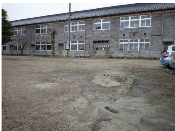
Fig.14 Damage of school building and markings of sand boiling in Osaki
