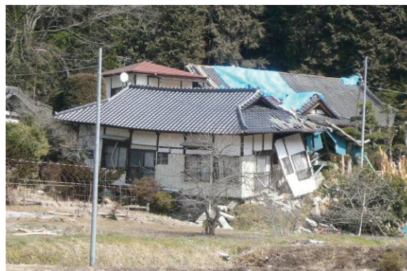
Fig. 6 Collapse of wooden house with high stone foundation
