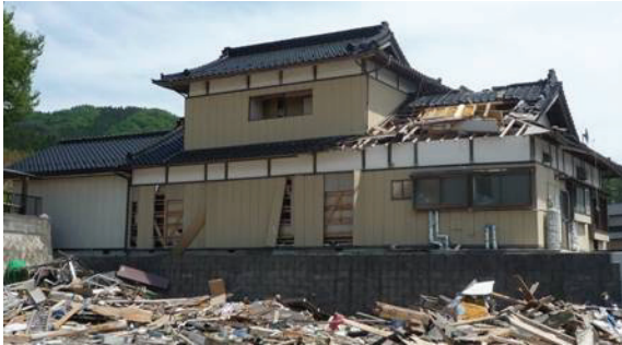
Fig. 46 Wooden house that avoided being carried away even with flood damage up to the 1st floor roof
