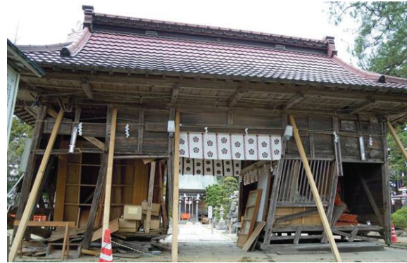
Fig.17 Severe damage to the gate of a shrine in Osaki
