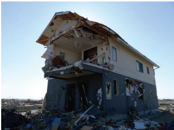
Fig. 26 Wooden building escaping complete devastation
