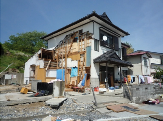
Fig. 43 Wooden house intact with 7m wave depth
