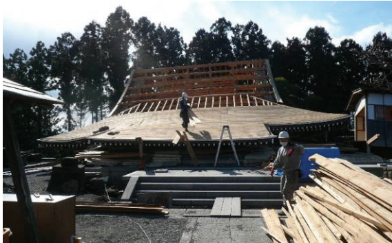
Fig.16 Collapse of the main building of temple in Takanezawa
