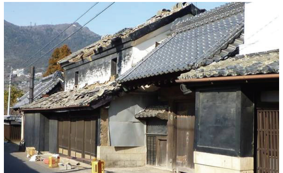
Fig.11 Damage of three storehouses with heavy mud walls
