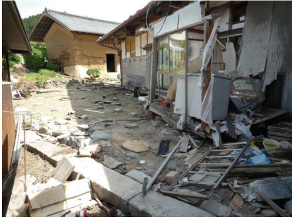
Fig. 49 Survived old house which was rotated
