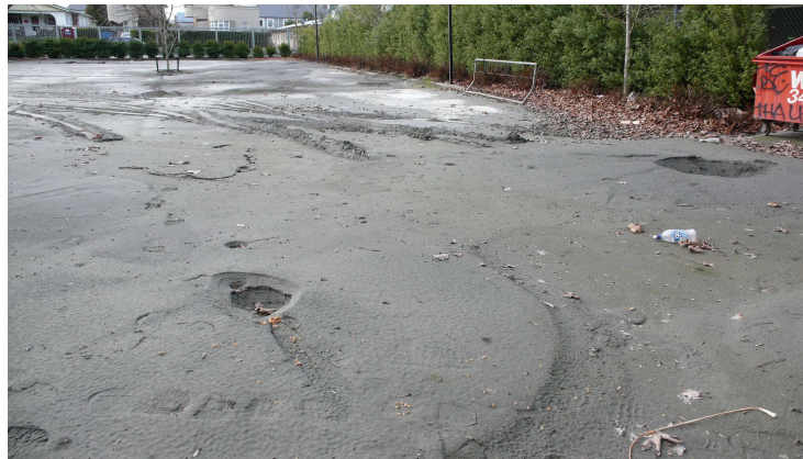
Fig. 2 Silty sand liquefaction at central business district of Christchurch during 2010-2011 Christchurch Earthquakes, New Zealand.
