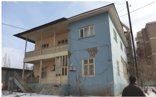
(a) Damage of adobe house
