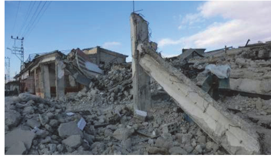
(b) Collapse of an industrial building
