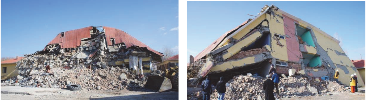
(a) West side of view (b) East side of view Photo 4 Overview of building
