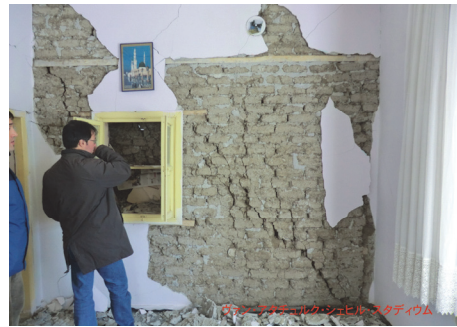
(b) Out of plane failure
