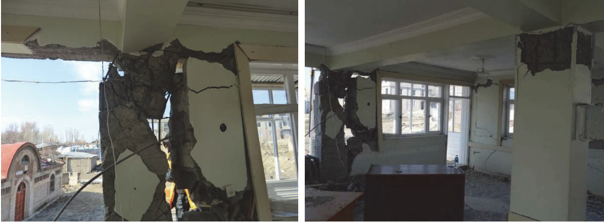
(a) West side column failing in shear (b) Column flexural yielding at the top Photo 2 Details of damaged columns
