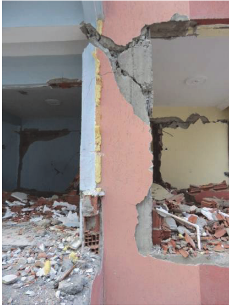
(a) shear failure of south side column of Building A (damage level V)
