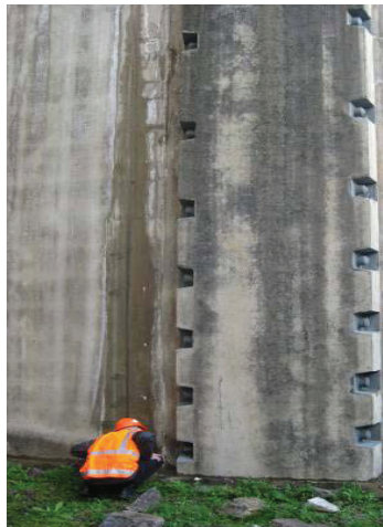
Fig. 4: No.1 Reservoir – leaking vertical wall joints.
