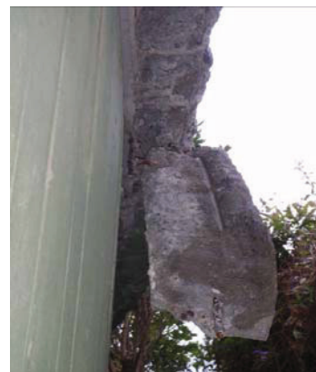
Fig. 7: Failure of roof overhanging nib.
