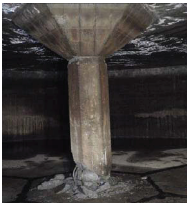
Fig. 6: Clifton 3 – internal column failure.
