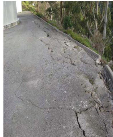
Fig. 5: Access road – cracking and slumping.
