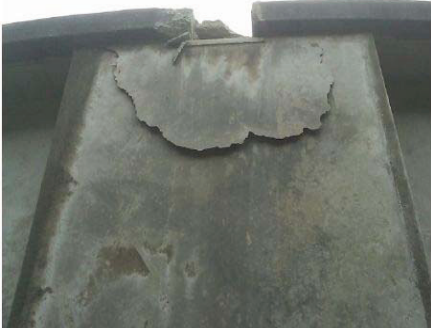
Fig. 8: Upper Balmoral – concrete shear failure at pilaster locations due to roof beam impact.
