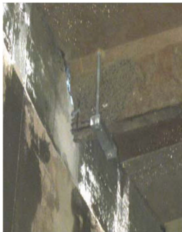
Fig. 3: No.1 Reservoir – significant roof damage.
