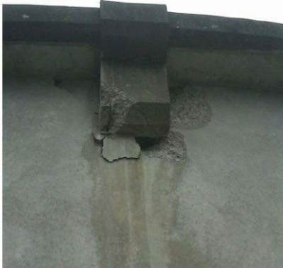
Fig. 9: Upper Balmoral – concrete damage at roof beam wall support.
