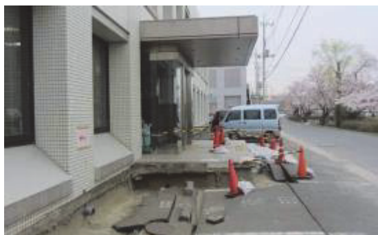
Photo 2 The ground in front of Katori Health Center subsided, and a depression of about 50 cm was created. (Sawara, Katori)
