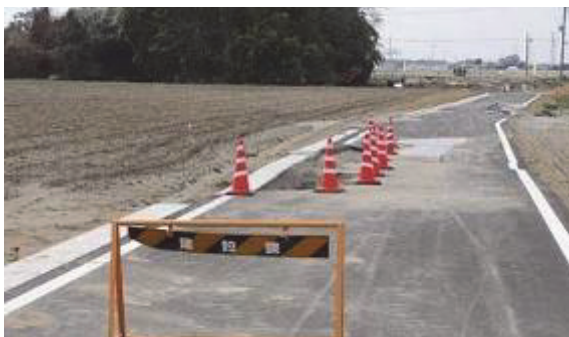
Photo 5 Sand boils and subsidence (Yoshino, Joso)
