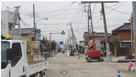
Photo 3 Large-scale liquefaction occurred, and many telephone poles became slanted. (Fusa, Abiko)
