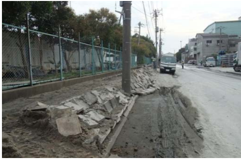
Photo 3 Heaving of a footway at Takahama, Ichikawa City
