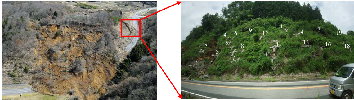
Fig. 11 A disturbed natural slope adjacent to the coherent landslide mass. The numbers for the ground anchors were marked for the reference to be used in future.
