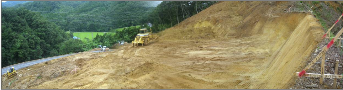
Fig. 8 Panoramic view of the landslide mass, re-profiled to an apparent stable configuration for the purpose of road construction.
