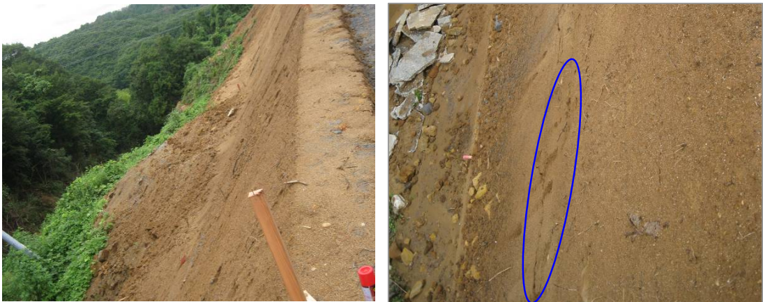
Fig. 9 Embankment of the road constructed on the landslide mass (left photo). Small scale cracks were observed near the base of embankment even during construction (right photo).
