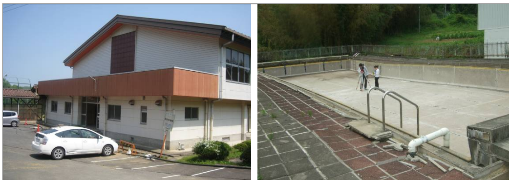
Fig. 12 Idosawa Fault passing under the gymnasium building (left photo) and swimming pool (right photo) of Tabito Junior High School, tilting and deforming the structures ( 36^{\circ}57'52.2'' , 140^{\circ}42'10.0'' )
