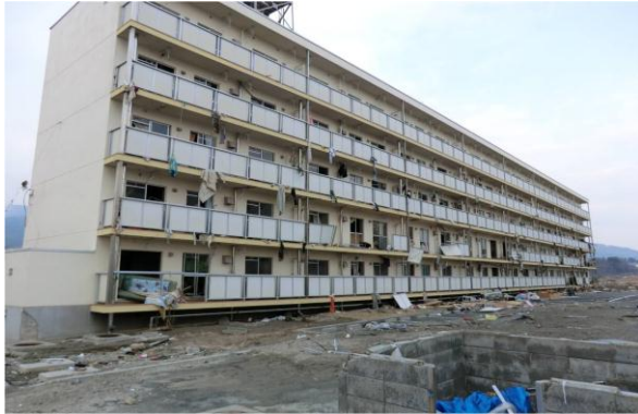
Figure 1 Survived a Five-story Concrete Building at Rikuzentakada, Iwate Prefecture in Japan(2011)
