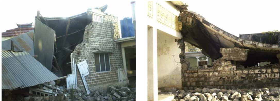
Fig. 5 Girls Degree College Rawalakot (left photo) and Boys Degree College Hajira (right photo) were totally collapsed during the earthquake. The structural system for both the buildings was load bearing stone masonry walls with different roofing system (Photo by Kazmi, 2006)
