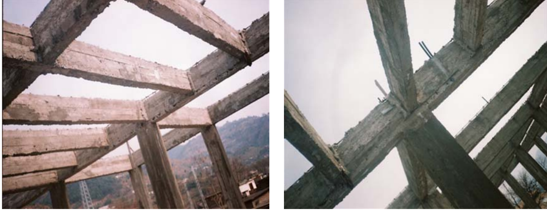
Fig. 8 A typical example of reconstruction for concrete frame structure (Photos by Kazmi, 2007).
