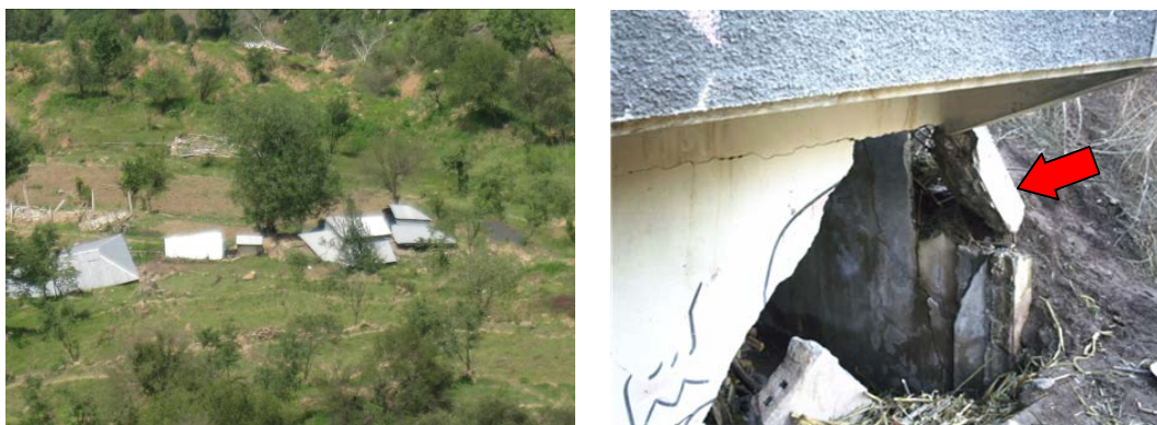
Fig. 4 Houses collapsed during the Kashmir earthquake with their rear walls damaged by increased earth pressure from the hill slope.
