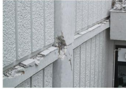
Photo 4 Crack in the 3 rd floor shear wall
