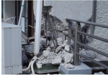
Photo 3 Heavily damaged southeast corner column base
