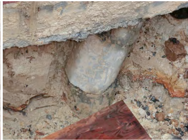
(b) Break-off and horizontal slip at pile top
