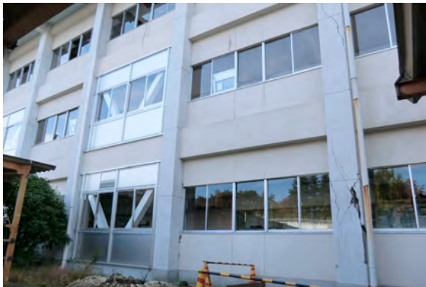
Photo. 3 Shear failure of column adjacent to unit bay strengthened by steel-braced frame
