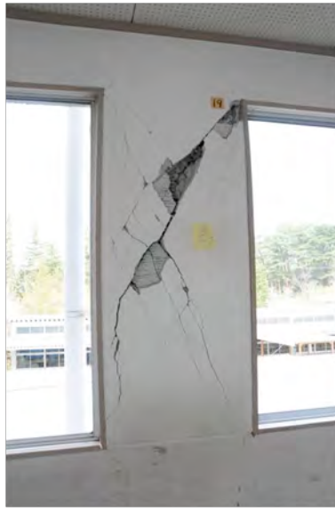
Photo. 6 Shear failure of C-8 column at second story
