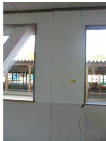
Photo. 9 Shear cracks of C-14 column at first story
