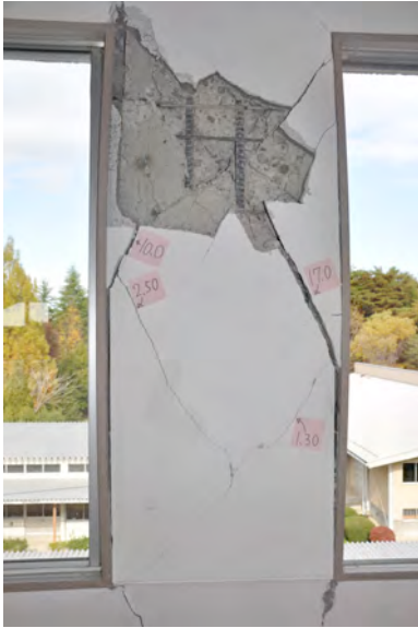
Photo. 5 Shear failure of C-13 column at third story
