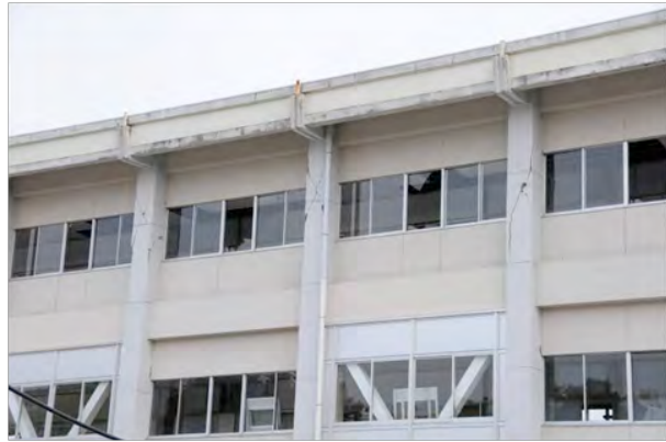
Photo. 2 Shear failure of columns in C frame at third story
