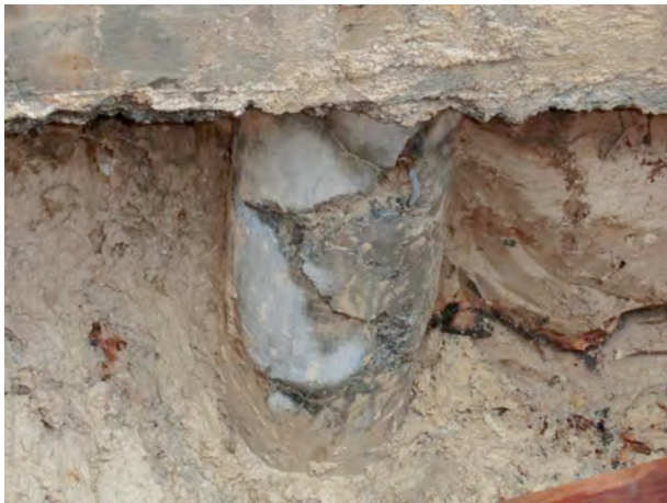
(a) Shear failure and bar buckling
