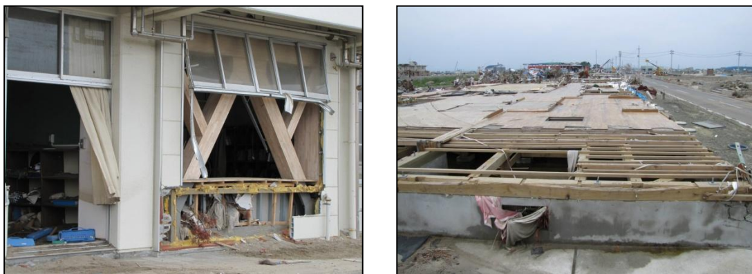
Fig. 5 Retrofitted school building (left) in Arahama Ward (Sendai) provided vertical shelter to the devastated community, where virtually no wooden structures remained (right) (Pierepiekarz)
