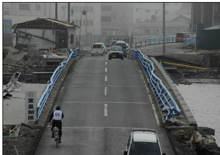
Fig. 6 Functional low-profile vehicle bridge in Ishinomaki City. Note damage from tsunami to leading edge of bridge walkway and guardrail on the left side of the photo (Swanson)
