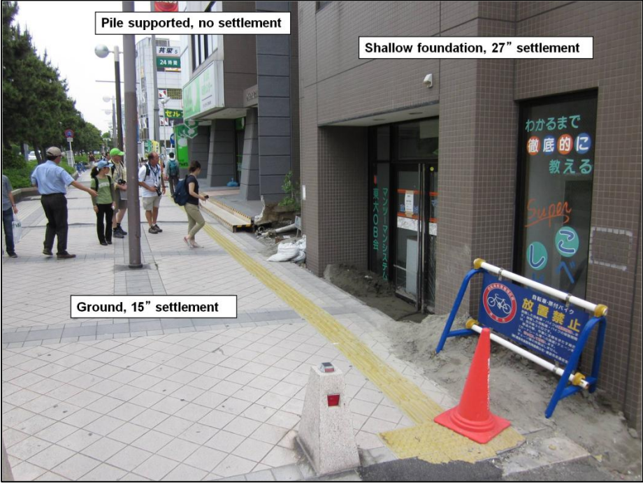
Fig. 3 Performance differences between adjacent buildings supported on piles versus shallow foundations in Urayasu City (Lindquist)
