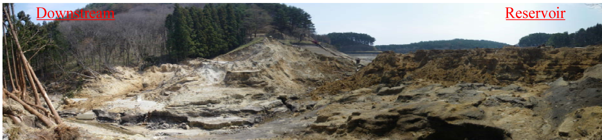
Photo 3 Breached dam body of large dam from left side (April 15 th at 37.302465, 140.195223)
