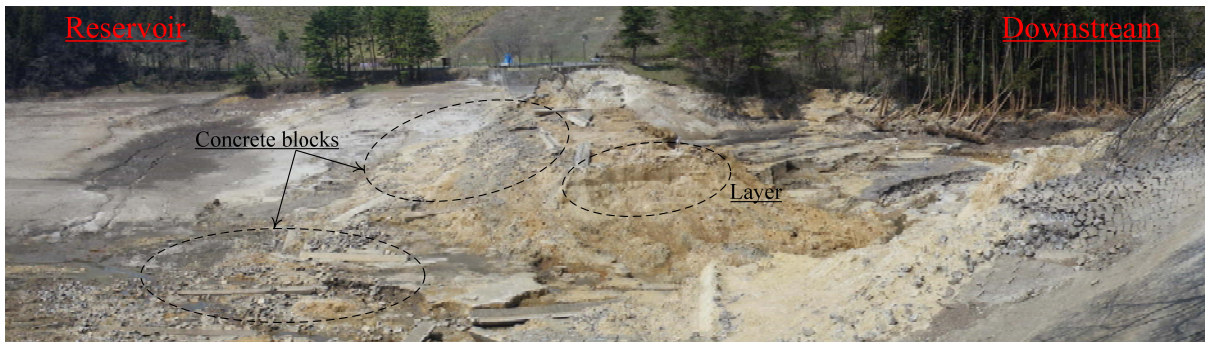
Photo 2 Breached dam body of large dam from right abutment (April 15 th at 37.301265, 140.195401)
