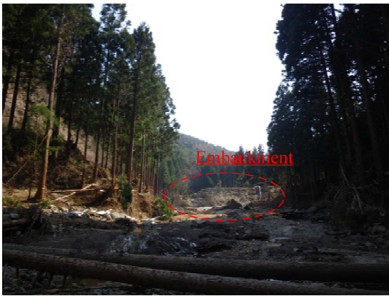
Photo 6 Breached road embankment (April 15 th at 37.305036, 140.198236)
