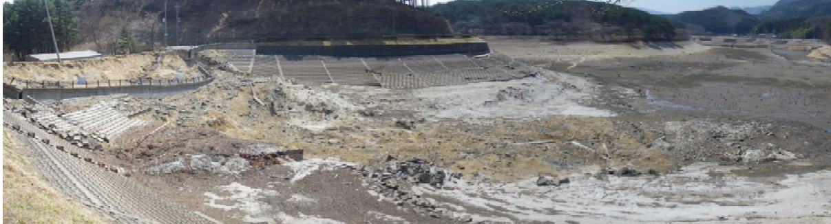
Photo 1 Sliding failure of small dam (April 15 th at 37.299778, 140.195348)
