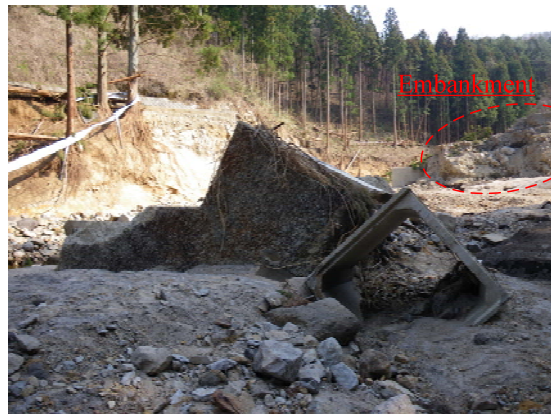
Photo 7 Washed out box culvert (April 15 th at 37.304499, 140.197989)
