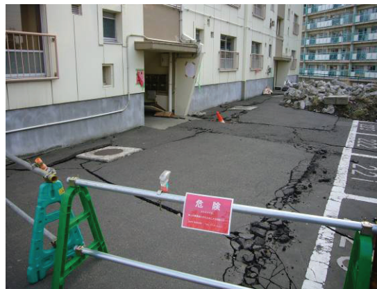
Photo 4 Damage of the ground around the apartment
