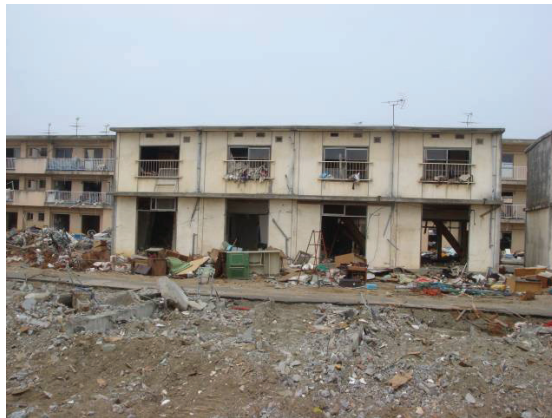
Photo 11 Mass production type public apartment building damaged by tsunami in Natori
