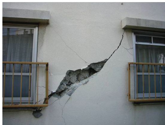
Photo 2 Shear failure of the bearing wall of the first floor at east side
