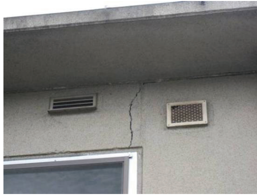
Photo 9 Crack at vertical joint between bearing wall and hanging wall
