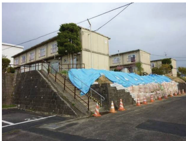
Photo 8 Mass production type public apartments and damage of the retaining wall
