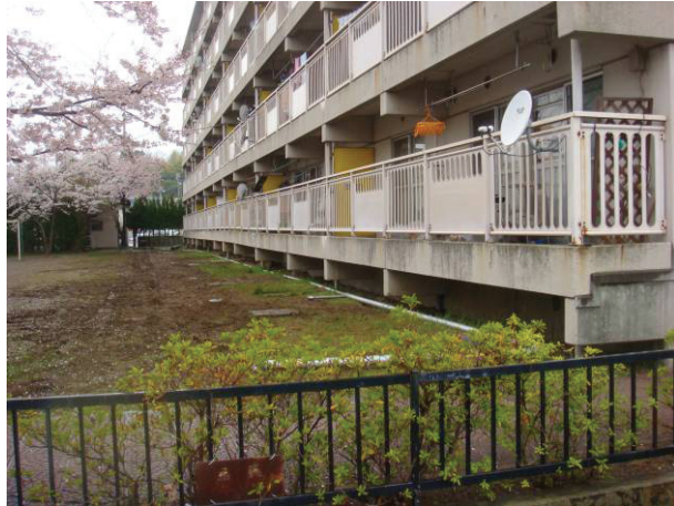
Photo 6 View of ground subsidence around d-apartment
