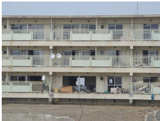
Photo 12 WPCa PS apartment building damaged by tsunami in Natori
