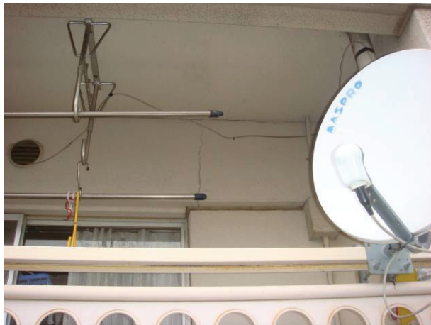
Photo 7 View of the crack at the beam of 2 nd floor of d- apartment
