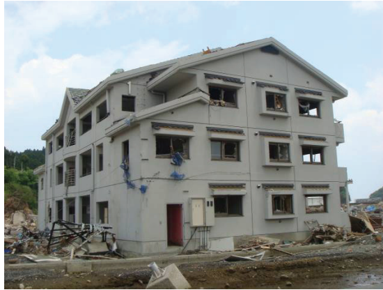
Photo 13 WRC apartment building damaged by tsunami in Minami Sanriku
