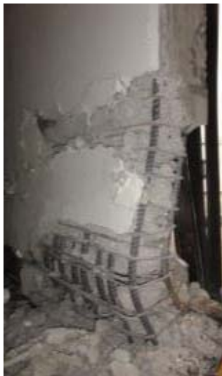
Figure 3a Wall failure in 2011 Christchurch earthquake (Elwood, 2011)
