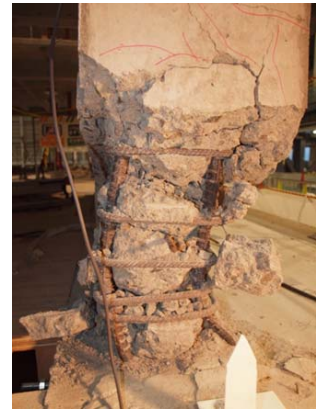
Figure 7b Wall damage
