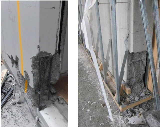
Fig. 5 Buckled and fractured bars in lightly reinforced slender RC shear walls.
