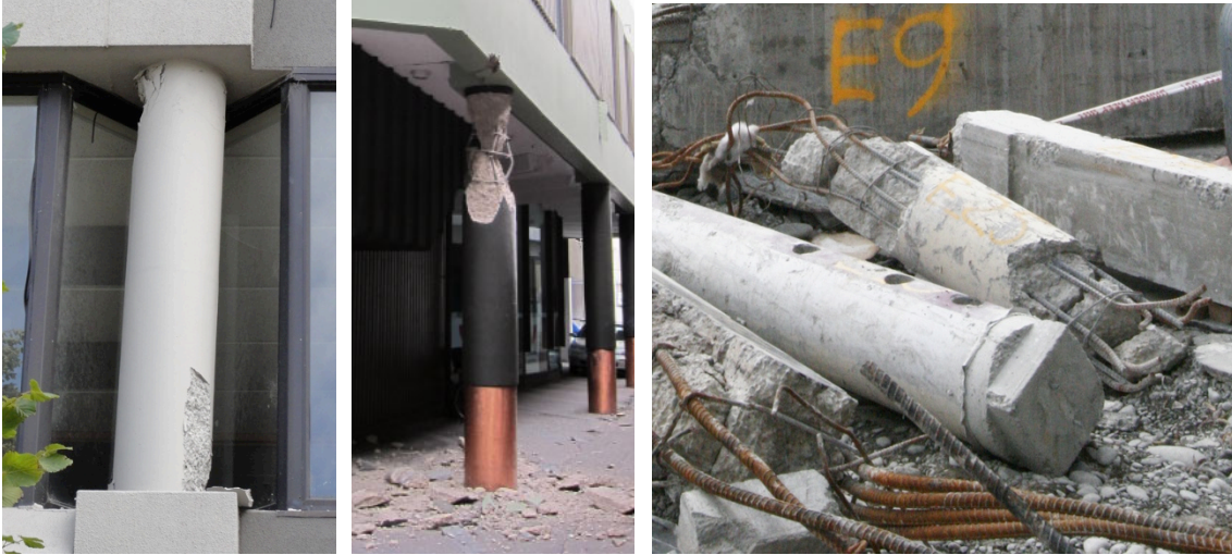
Fig. 10 Damage to gravity columns
