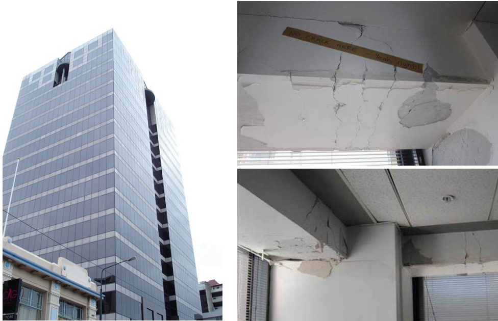
Fig. 3 Beam cracking in 22-story RC moment frame (precast emulating cast-in-place)
