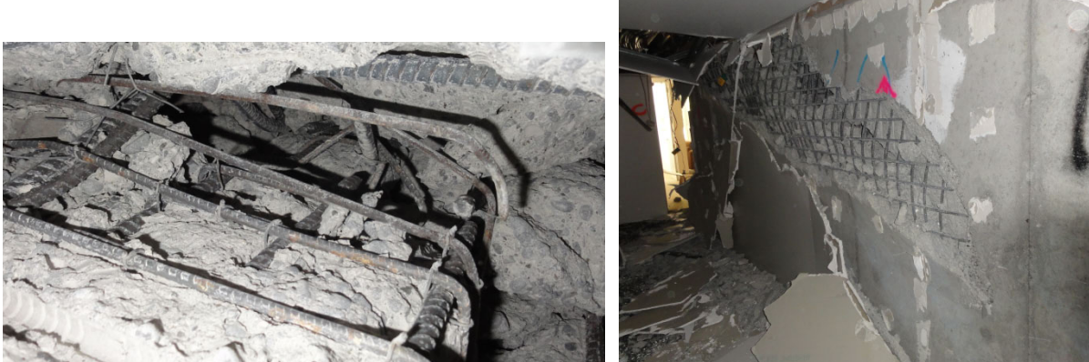
Fig. 6 Boundary bar fracture and web crushing in modern 8-story apartment building.
