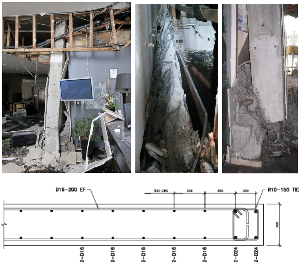
Fig. 7 Crushing and out-of-plane movement of shear wall in 22-story Hotel Grand Chancellor (Middle and right photos from Dunning and Thornton (2011))
