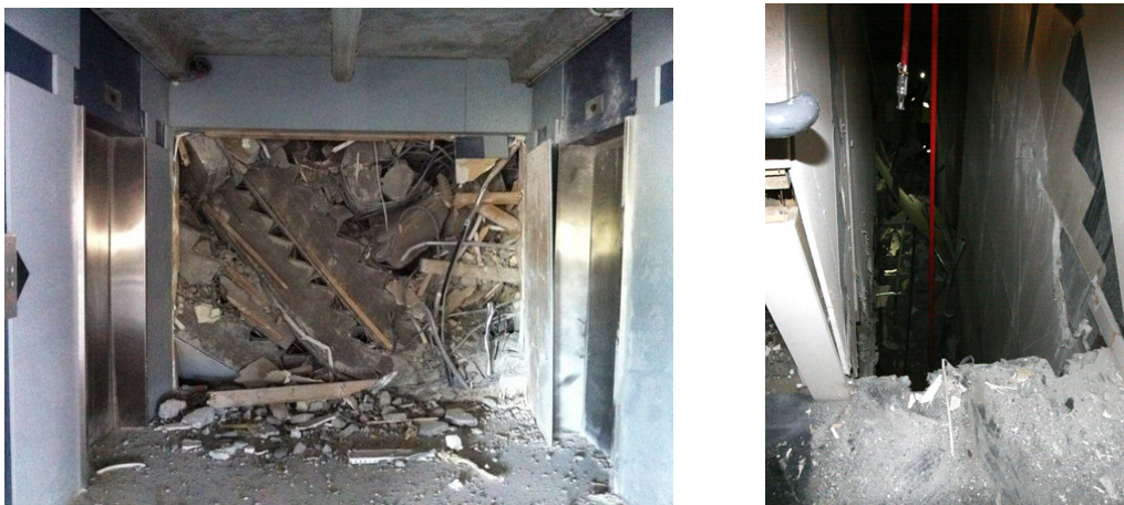
Fig. 8 Collapse of precast stairs
