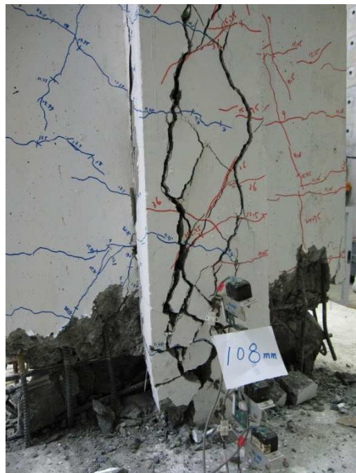
Fig. 11 Final failure state of the specimen S5 when the drift ratio reaches to 6%
