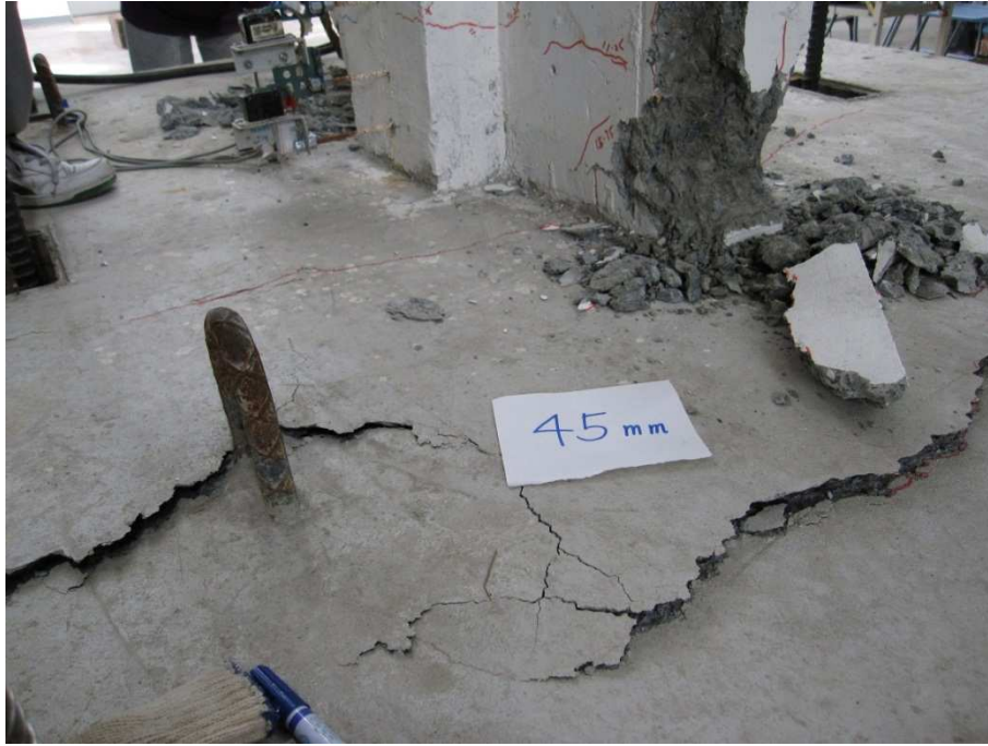
Fig. 10 Damage state of the footing of the specimen S4 when the drift ratio reaches to 2.5%
