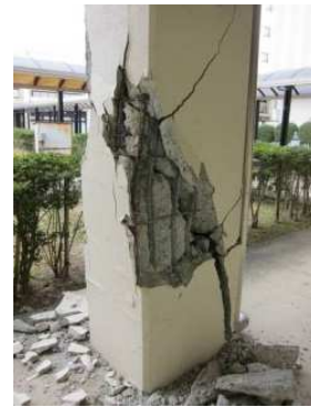
Fig.7 After 7 th of April aftershock earthquake
