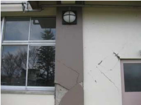
Fig19 Shear Crack in side walls. Building (B)
