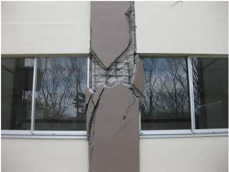
Fig18. Shear failure in column. Building (B)
