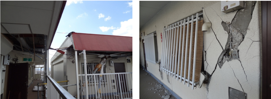
Photo 2 Gap between the buildings at the 14 th floor and damaged non-structural wall
