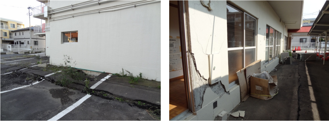
Photo 3 Damage around the foundation and damaged non-structural wall at the first floor
