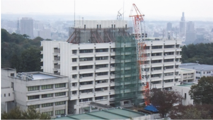
Photo 1 General view of the building after tentative strengthening of the damaged penthouse
