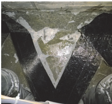
Photo 5 Unstuck tapes Floor 5 Frame 12 Beam I-J
