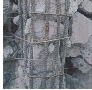
Photo 16 Column of the penthouse after the earthquake
