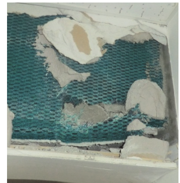
Photo 7 Broken fibers Floor 7 Frame 11 Beam I-J
