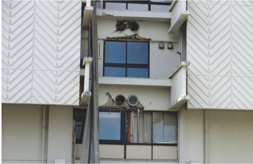
Photo 12 Coupling beams damaged around openings
