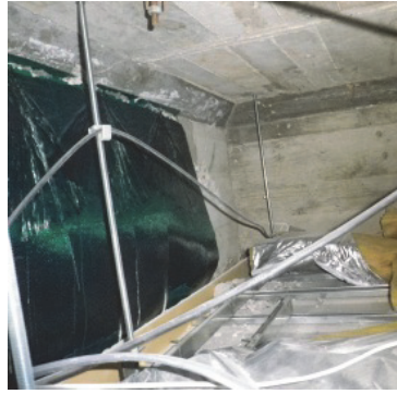
Photo 9 Anchorage failed Floor 6 Frame 12 Beam I-J
