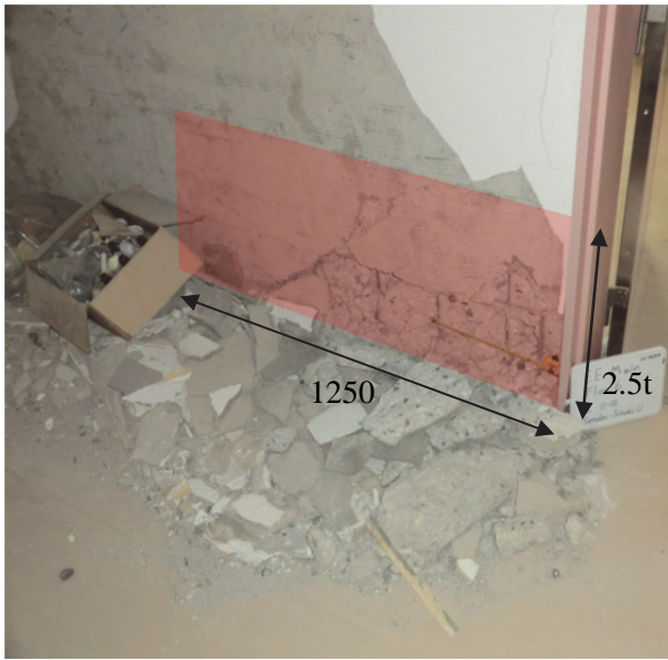
Photo 13 Compressive failure Floor 6 Frame I between frames 11-12
