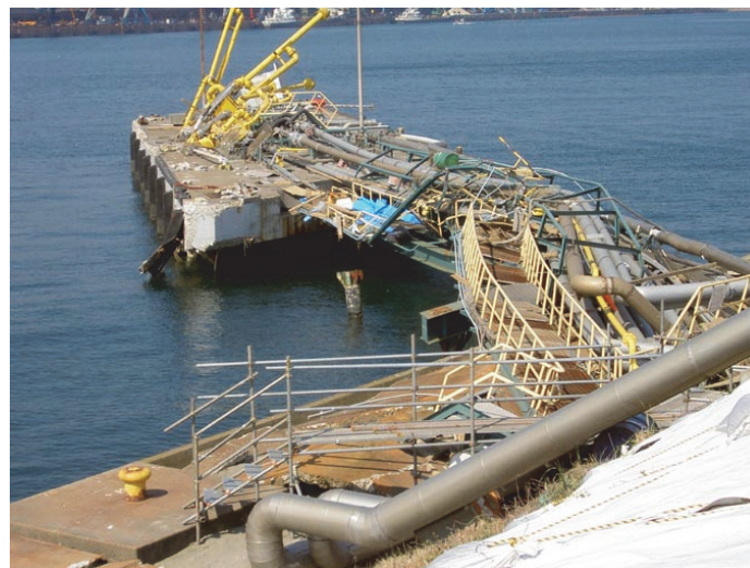
Photo 3 Berth collapsed by an oil tanker strike
