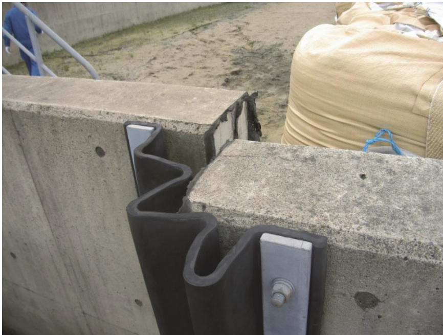
Photo 9 Fracture of wall joint of the dyke with rubber sheet protection
