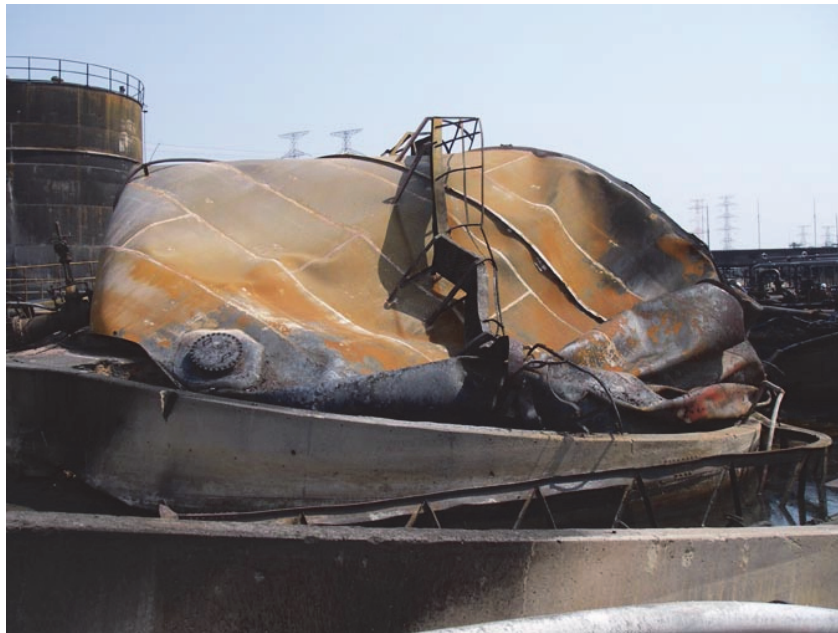
Photo 5 Burned-out gasoline tank
