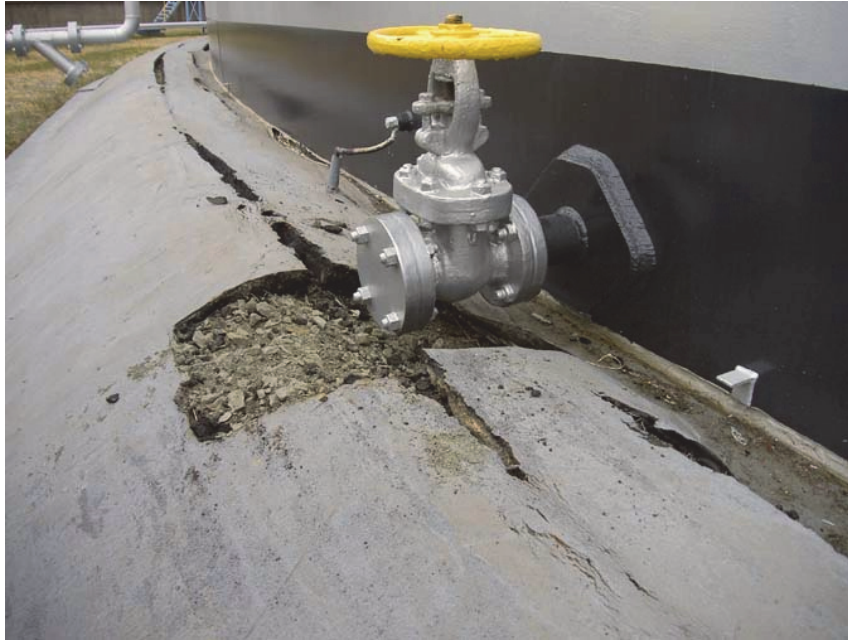
Photo 8 Tank settled because of liquefaction around the foundation
