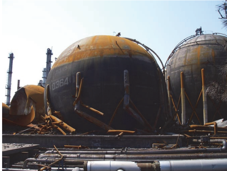
Photo 6 All legs of the LPG tank collapsed and buckled by the earthquake
