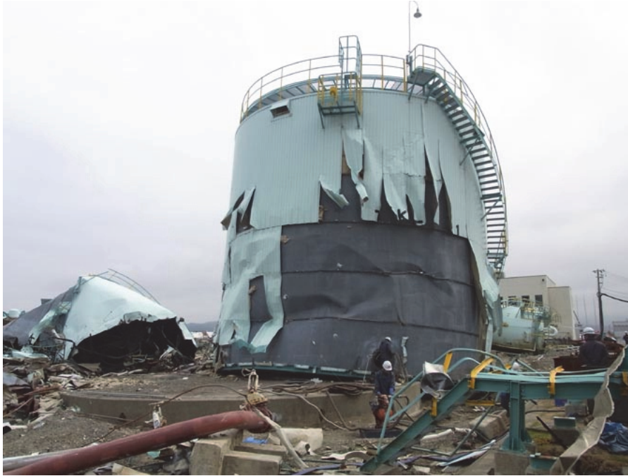
Photo 14 The tank of which the shell plate buckled and the heat reserving materials tore off
