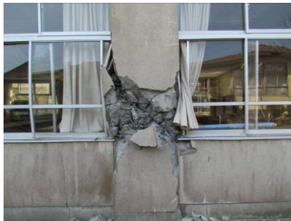
Fig. 3 Shear failure of the first story column at north frame of Building “A”
