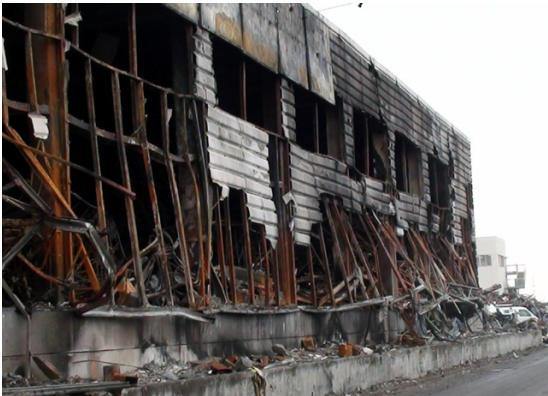
(a) The first floor was destroyed by the tsunami and fire
