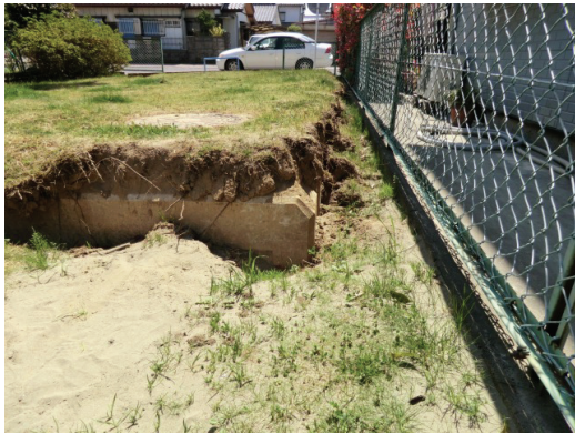
Figure 18 Water tank uplifted by liquefaction
