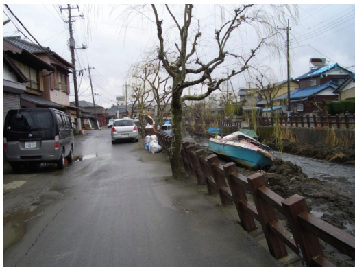
Figure 6 Damage to the revetment along Ono River
