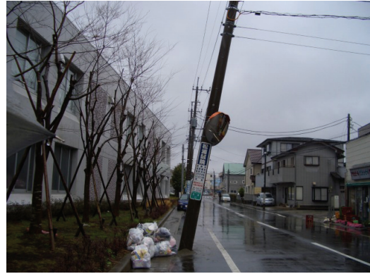
Figure 3 Leaning power pole
