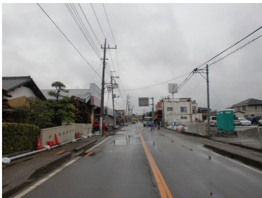
Figure 20 Liquefaction in Miyako
