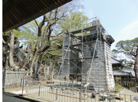
Figure 29 Damage to a stone structure
