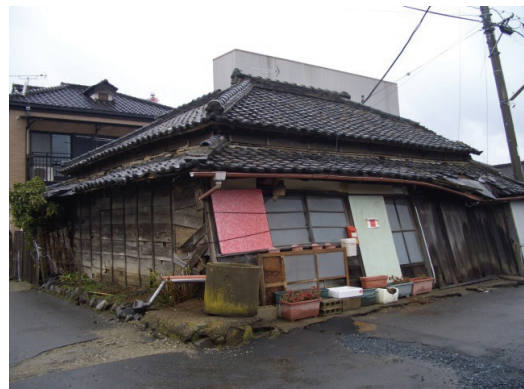
Figure 7 Timber house damage from liquefaction
