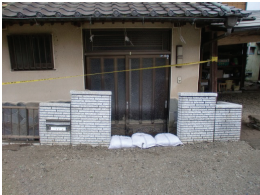
Figure 24 Settling of a timber house due to liquefaction
