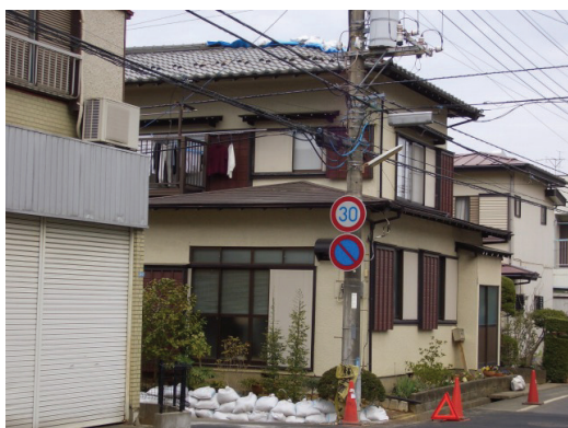
Figure 32 Settling of a timber house
