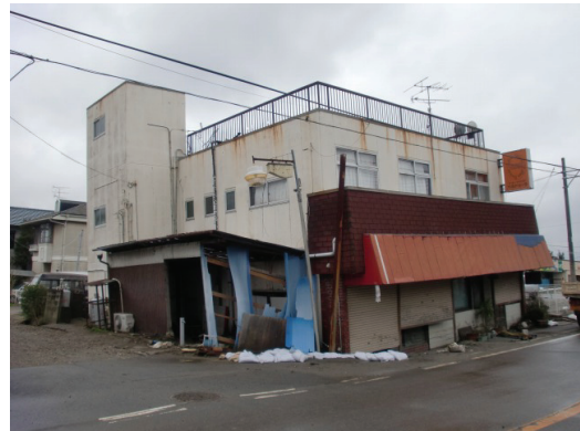
Figure 25 Inclination of a building due to liquefaction
