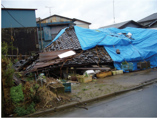
Figure 8 Collapsed timber house near the Ono River Drainage Pump Station
