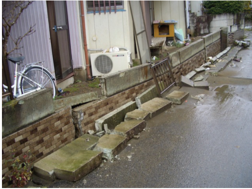
Figure 2 Damage of a masonry garden wall
