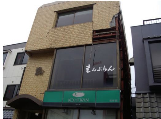
Figure 27 Fallen exterior walls
