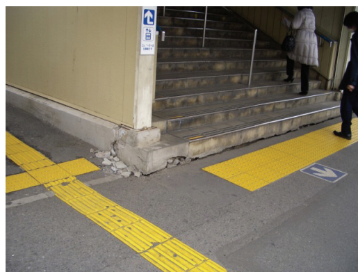
Figure 33 Damage to a column base of the stairs in Keisei-Sakura Station.
