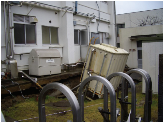
Figure 4 Damage of a tank by land subsidence
