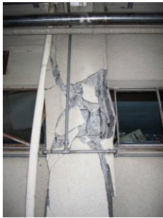
Fig. 16 Shear failure of column
