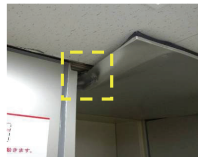
Fig. 22 Expansion joint deformation
