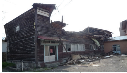
Fig. 8 Collapse of 2 nd story
