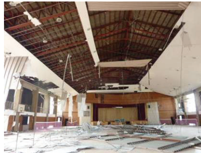
Fig. 13 Dropping of ceiling
