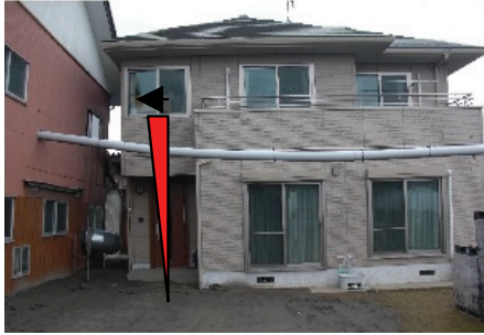
Fig. 23 Tilted house by liquefaction
