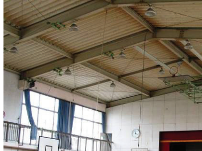
Fig. 10 Rupture of roof braces
