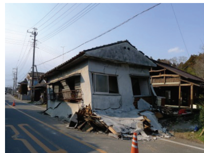
Fig. 6 Collapse of 1 st story
