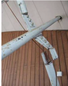
Fig. 9 Rupture of brace joint
