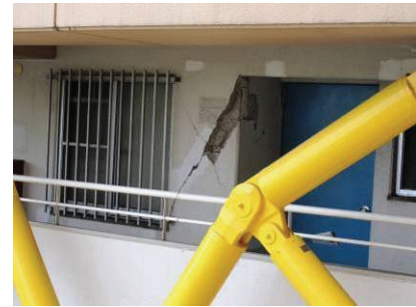
Fig. 18 Damage of retrofitting
