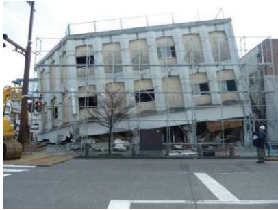
Fig. 14 Collapse of soft 1 st story
