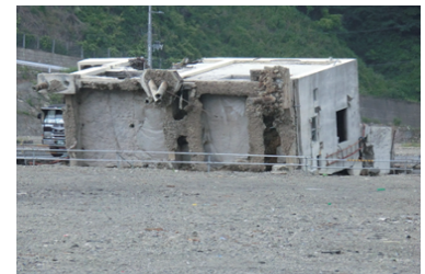
Figure 2. Overturned building due to tsunami
