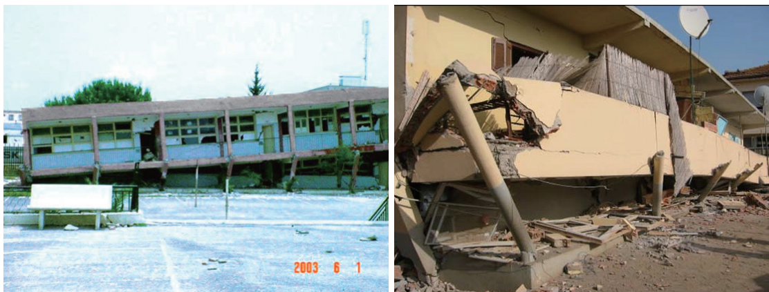
Fig. 1 Destroyed schools in Algeria during the seismic event of 2003. Source: EERI Learning from Earthquakes Reconnaissance Report
