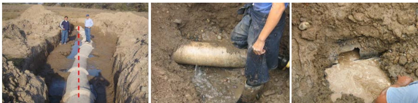
Figure 1. Damage to water distribution pipelines following the 2007 Pisco earthquake in Peru.
